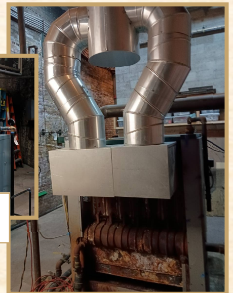
New Boiler vs. Corroded Boiler
